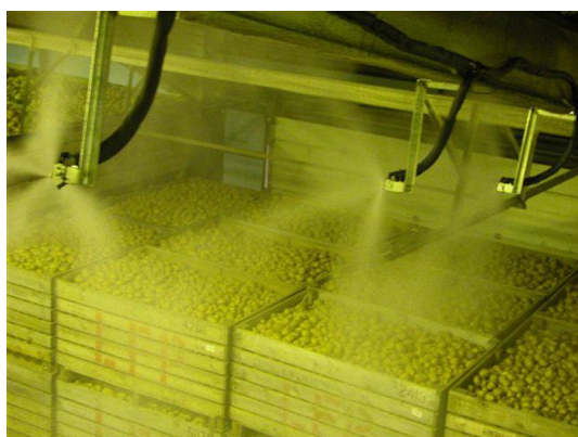
Figure 7. Packed potatoes treated by using Pimi's SpuDefender installation at a Branston farmer site in the UK, October 2008 (reproduced with permission from Ref. [48], with kind permission).
