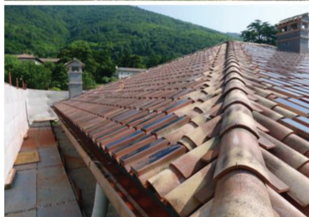
Figure 4. A 6 kWp solar array in PV bent tiles comprising the rooftop of an early 1900s villa in Valdobbadiene, Italy (Photos reproduced with permission, courtesy of Industrie Cotto Possagno).
