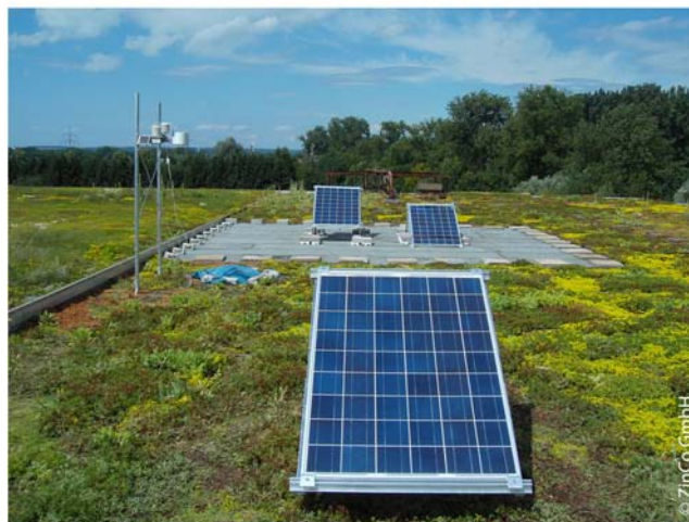
Figure 7. The PV modules tested during one solar year installed on bituminous membrane and on a green roof (photograph courtesy of ZinCo GmbH).
