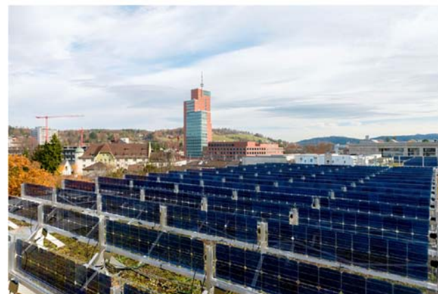
Figure 4. Aerial (top) and later (bottom) view of the 909 kW PV array on the rooftop of a building of Zurich University of Applied Sciences in Winterthur (photograph courtesy of T. Baumann and Zurich University of Applied Sciences).
